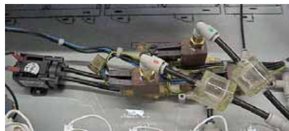
Water distribution incl. filters
